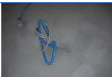
Bad workmanship Electric tubes in floating floor without insulating sleeve
