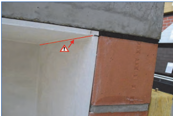
Figure 2.13. Detail of the acoustic strip below the concrete slab and on top of the wall. It is always important to cut the plaster at the junction between the brick wall and the concrete slab to avoid cracks (different thermal dilatation), but when using acoustic strips, it should be cut completely down to the acoustic strip and filled up with silicones to avoid a “vibration bridge”.
