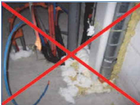
Figure 8.12. Example of problems related to piping system going through separating floor slab.
