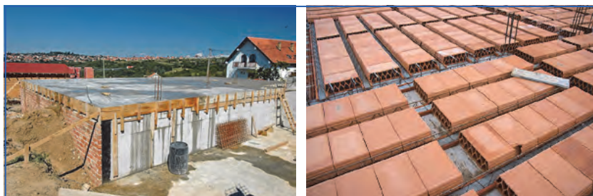
Figure 3.8. The most common floor slab designs: reinforced concrete (left) and brick system (right).
