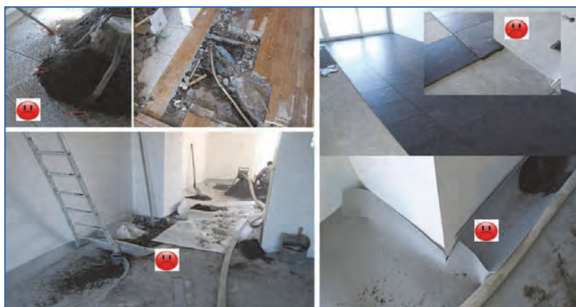
Figure 2.36. Bad execution of a mounting floor; sharp objects can puncture the elastic interlayer. Foils should have sufficient overlap and should be taped together. The against the wall upwards turned elastic interlayer should only be cut off after the tiling (if before, the tiles or the glue can make a hard connection with the wall, seriously diminishing the impact and airborne sound insulation of the floating floor).
