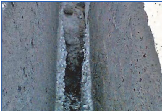
Figure 26.14. Casting waste between separated floor plates for row houses causing sound bridges.
