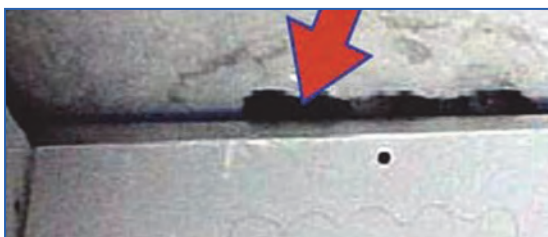
Figure 26.16. Holes not sealed.
