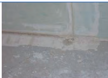
Bad workmanship Resilient layer on floor covered by plaster
