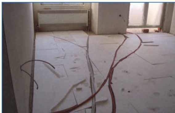
Figure 15.7. Typical error in workmanship – broken insulation.
