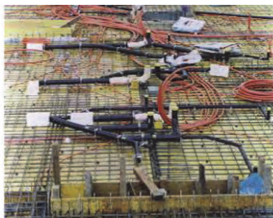
Bad workmanship Water pipes in concrete floor without insulating sleeve
