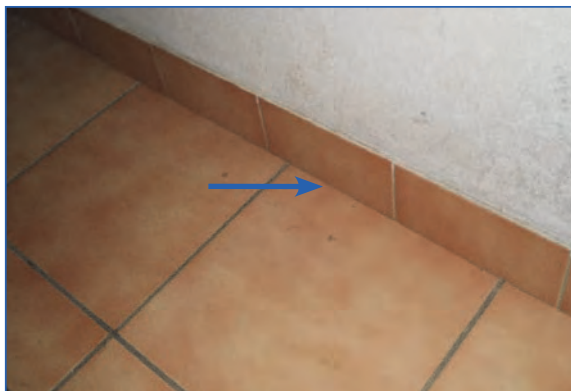
Figure 24.10. An example of a rigid contact of wall and screed via floor ceramics.
