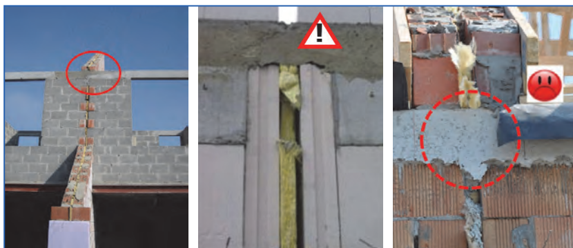
Figure 2.7. Hard connections (continuous floors, concrete beams but even small metal ties can largely reduce the sound insulation; the party wall loses its acoustic double wall behaviour and extra flanking transmission will occur.
