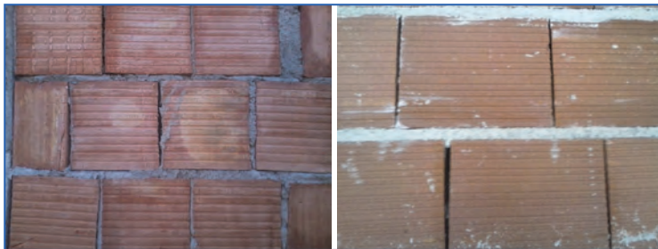
Figure 15.12. Typical errors in workmanship – vertical joints not filled with mortar.
