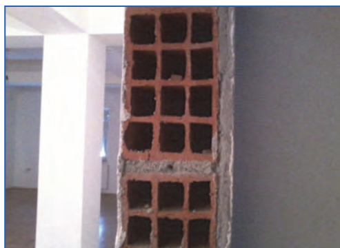
Figure 15.11. Typical errors in workmanship – irregular mortar layers.
