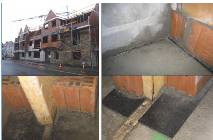
Figure 2.14. Application of acoustic strips below brick walls (party wall below) and concrete blocks (the elevator shaft). The acoustic strips (CDM, Sonic strips) have only a limited deformation (2 mm under the weight of the building, almost no creep in time).
