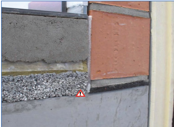
Figure 2.12. Detail of concrete slab with floating floor and acoustic strip (Sonic strip, Wienerberger – CDM). It is important to put a border resilient strip before executing the levelling screed to avoid a hard contact between the concrete slab and the brick wall!
