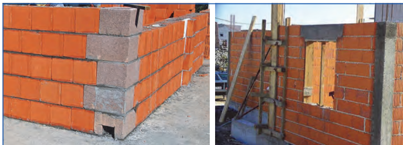
Figure 3.6. Anti-earthquake reinforcements done properly (left) and improperly (right).
