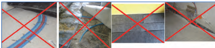
Figure 8.11. Example of problems related to floating floors.
