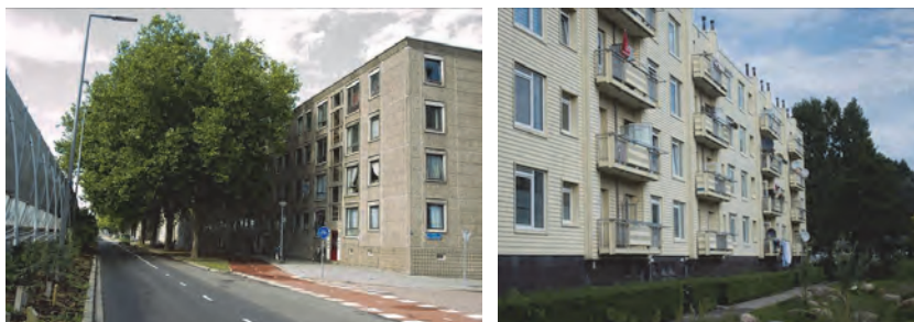
(Left) Porch houses built in the 50's and renovated in the 80's because of sound insulation of the façade and (Right) Porch houses also built in the 60's, renovated in 2010, with as main topic thermal insulation.
