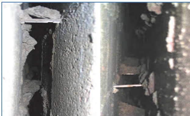
Figure 29.6. Example of poor workmanship in cavity separating walls, showing incorrect wall ties and also mortar being allowed to collect on ties (these provide strong acoustic bridges which weaken the sound insulation performance by 6 dB to 10 dB).
