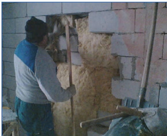
Figure 11.7. Stuffing the cavity with glass wool – a typical workmanship error of constructing double walls and furrings.
