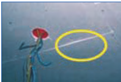
Figure 26.19. Wrong installation of resiliently suspended ceiling causing sound bridges, reducing the effect of the resilient mounting.
