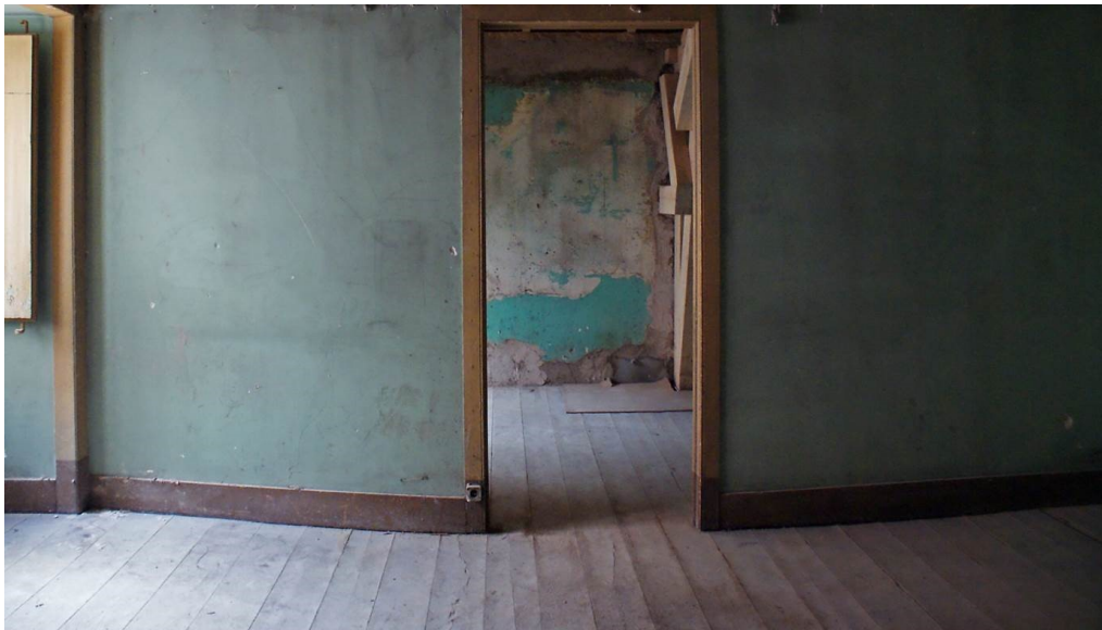
Figure 2: Excessive timber floor deflection and effect on the supported partition wall (Courtesy of NCREP).
