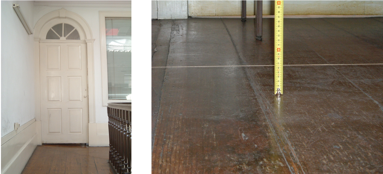
Figure 1: Jammed door due to excessive timber deflection and illustration of the deflection as deviation from a straight line (Courtesy of NCREP).
